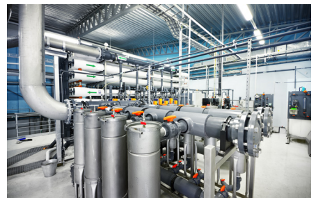
Water Pump Station
